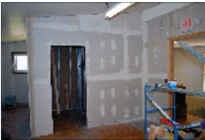
Above and to the left is the new closet at the head of the stairs.
